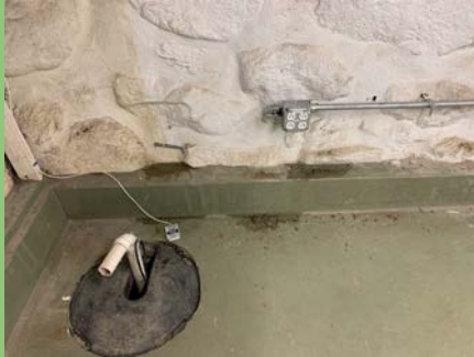
Basement water sensor
